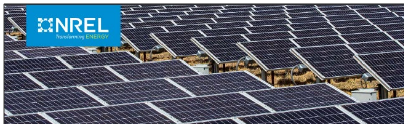
The 1MW photovoltaic array at the Flatirons Campus (FC) of the National Renewable Energy Laboratory (NREL). Photo by Werner Socarr, NREL 65307
