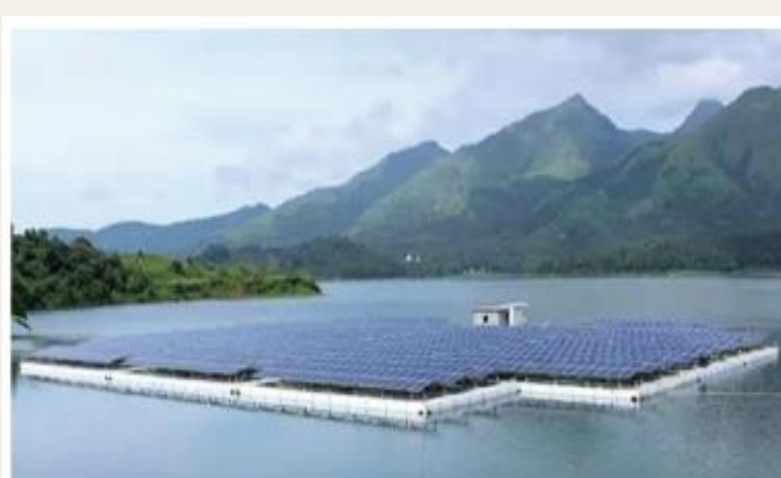
Fig. 3. A proof of concept implementation of a 500 KW FPV plant at Wayanad in Kerala [8]
