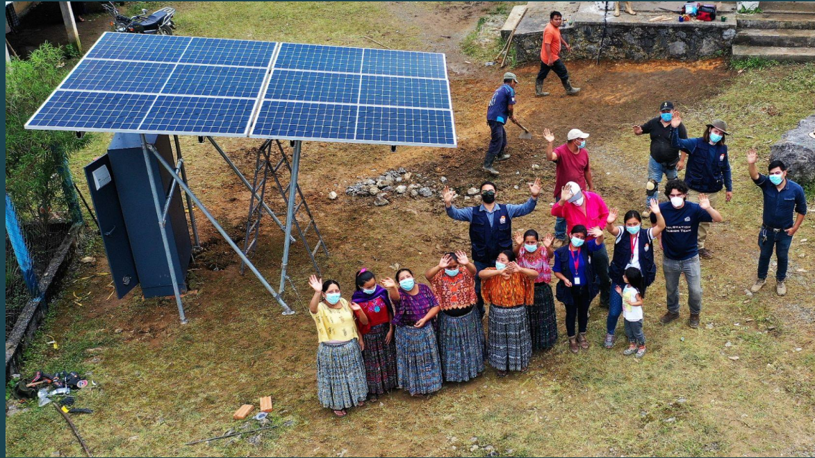
Digital Community Center installed by New Sun Road in San Antonio IV, Alta Verapaz, Guatemala
