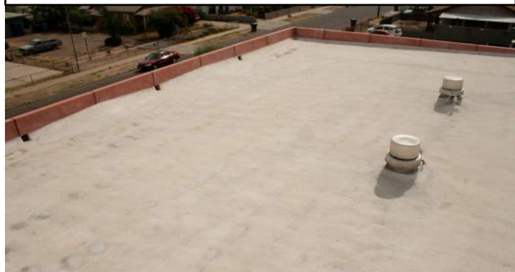
Photograph of the flat roof area showing the obstructions of the Fire Station building
