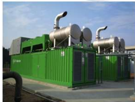
Fig 9. 10-ton/day Pyrolyzer and 800 kW CHP Modules in 40 ft. ISO Containers
